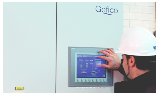
Control software for Gefico plant.
